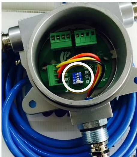
Dial switch inside Junction box
